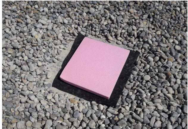
Figure 4: Insertion of the intermediate layer of XPS, underlaid with a protective layer of fleece (if necessary)
