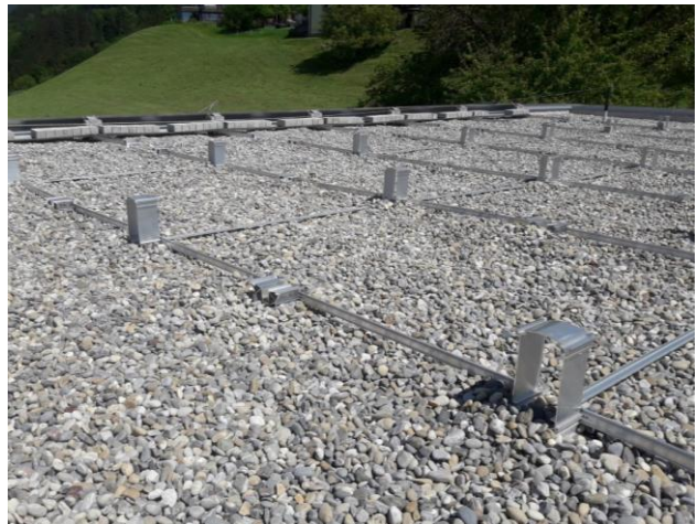
Figure 8: MSP-FR mounting system completely installed
