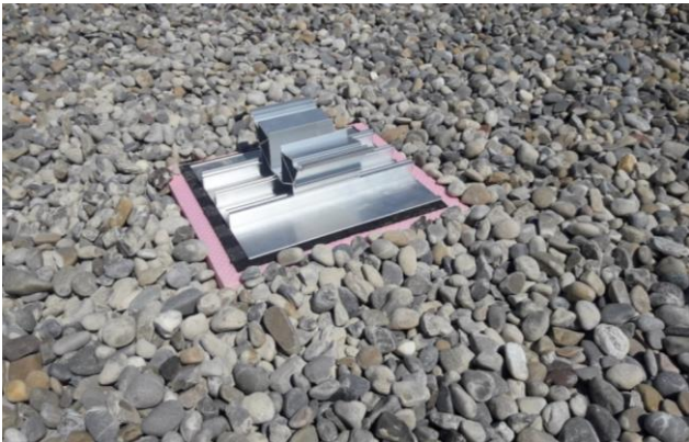
Figure 5: Placement of the base plate with support, fleece under the base plate
