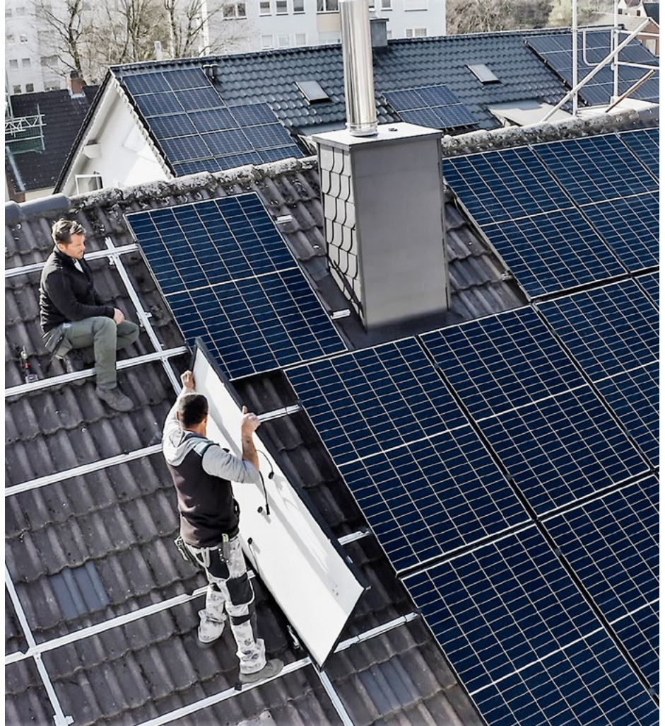
MSP-PR on-roof Ahlen (Germany)
