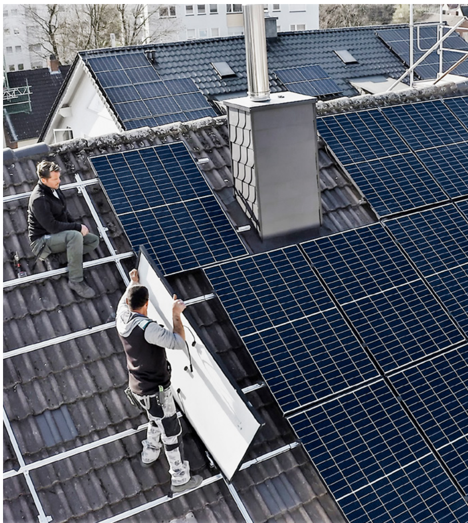
MSP-PR on-roof Ahlen (Germany)
